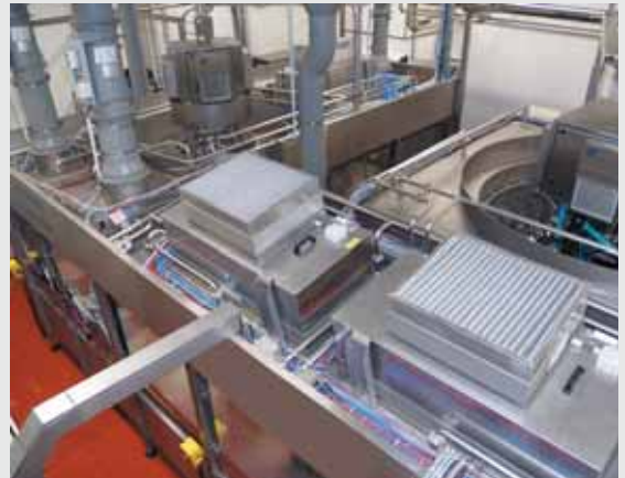
Supply air and return air system at aseptic filling machine
