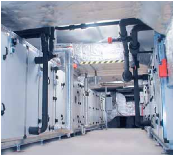
Central air-conditioning units for interior and exterior location
